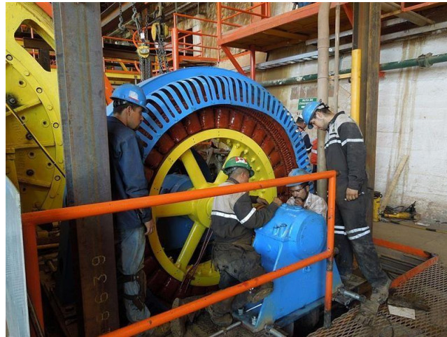
In ball mill in a mine ore process
