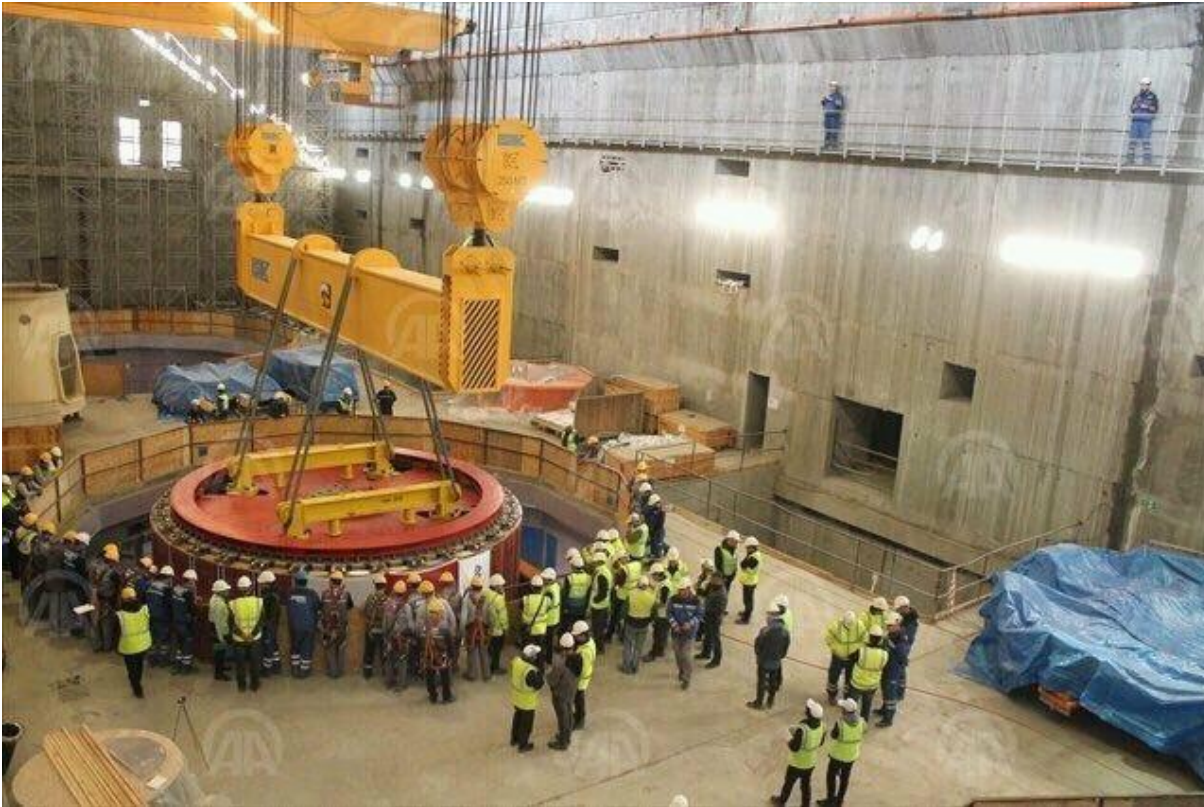
The rotor is being replaced inside the stator of a large synchronous generator in a hydro power plant
