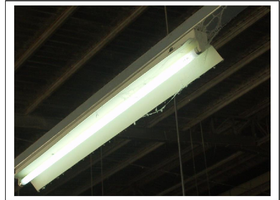
Figure 1: Here is a strip light covered in cobwebs and never cleaned. It is a waste of electricity costs and provides poor lighting for the workers.
