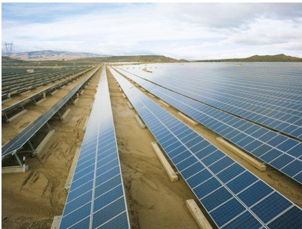
Arnedo Solar Plant, Spain
