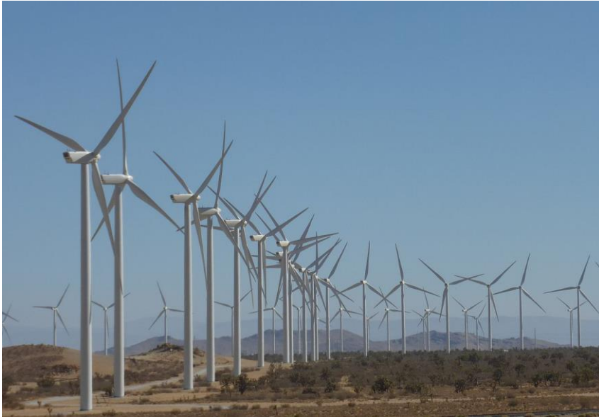
1020 MW wind power plant USA-California
