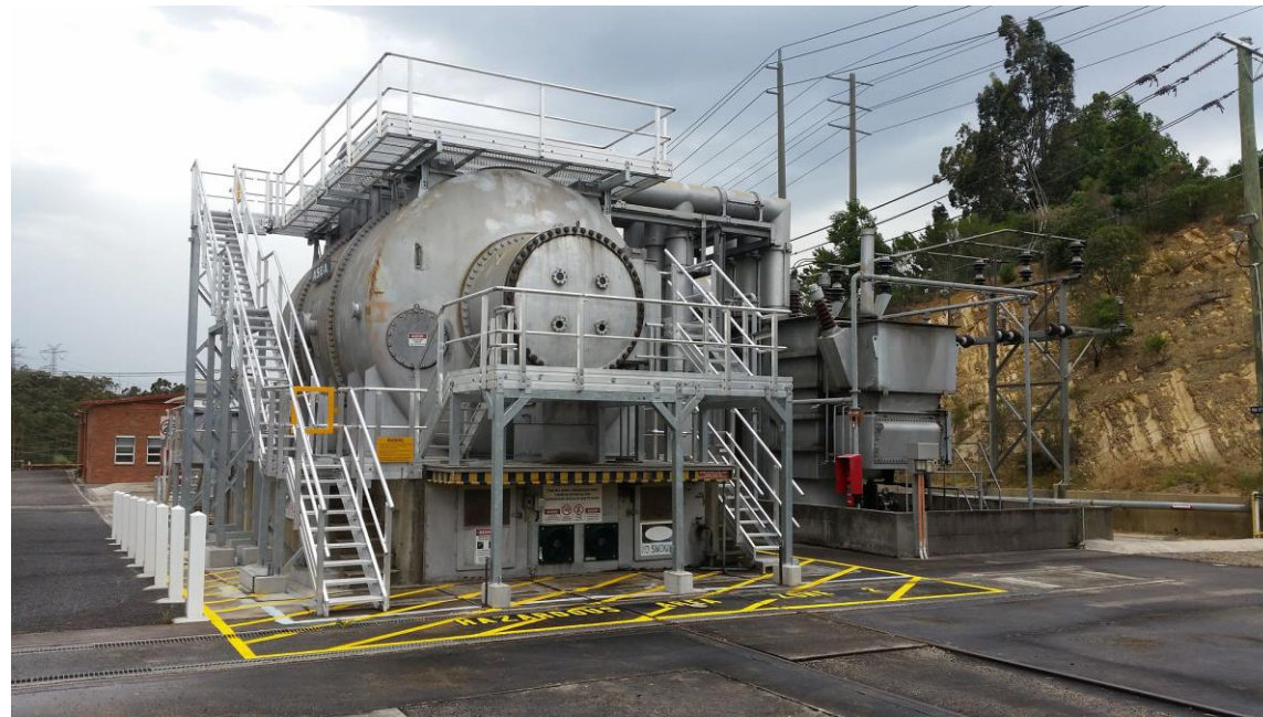
Synchronous condenser installation at Templestowe substation, Melbourne Victoria, Australia. Built by ASEA in 1966, the unit is hydrogen cooled and capable of three phase power at 125,000 kVA. Source Wikipedia.
